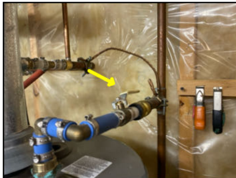
Location of the cold water shut off valve
