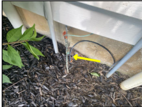
Location of the main electrical ground wire
