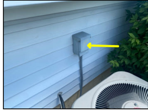
Location of the air conditioner disconnect
