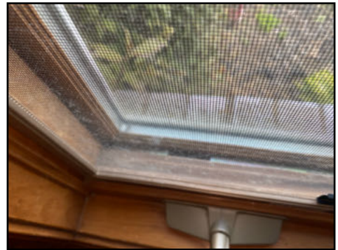
Window doesn't shut properly
