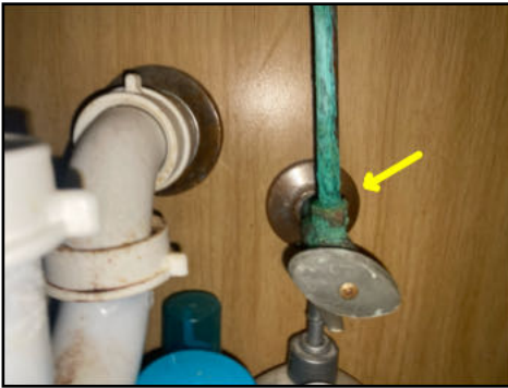
Corroded water line
