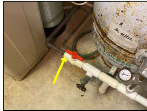
Location of the main water shut off valve
