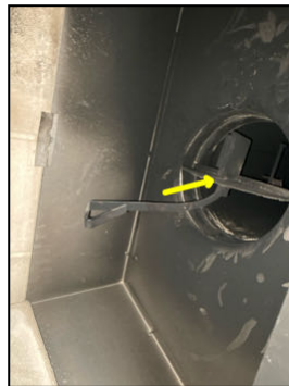
Missing damper clamp
