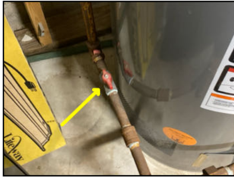
Location of the shut off valve
