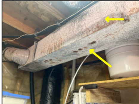
Ductwork is disconnected
