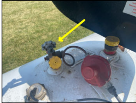
Location of the main propane shut off valve
