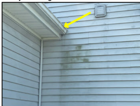
Missing kick out flashing
