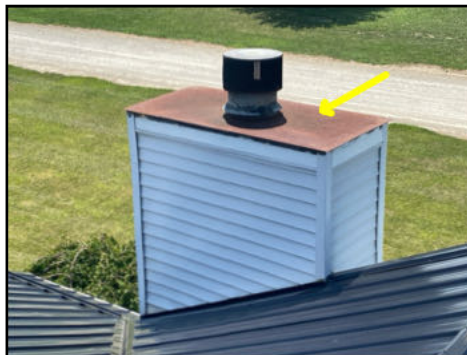
The chimney cap is slightly rusted but appears to slope properly
